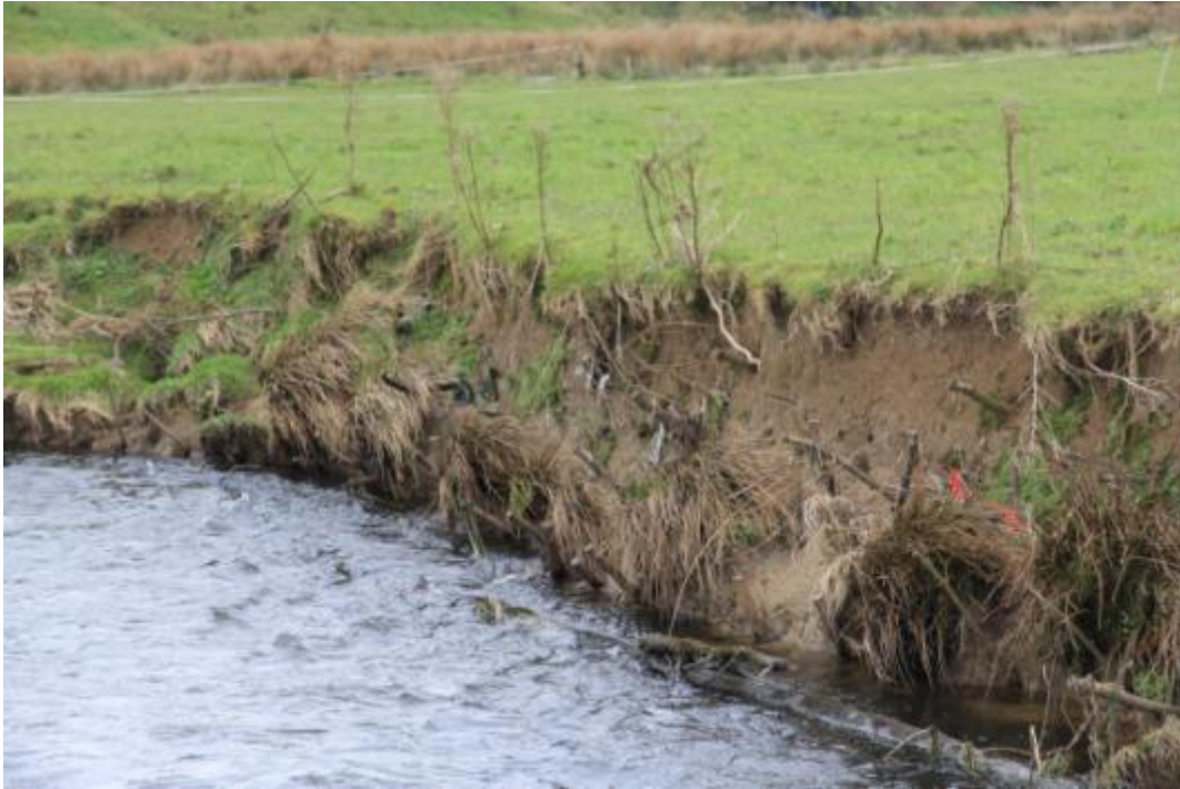
Willow stakes planted into high bank which did not take root and grow
