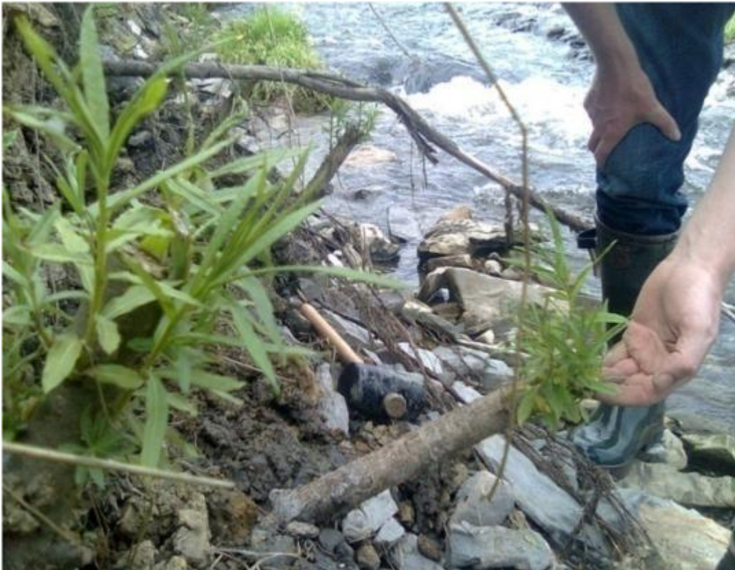
Sometimes the erosion was too quick for the stakes to root and protect the bank in time
