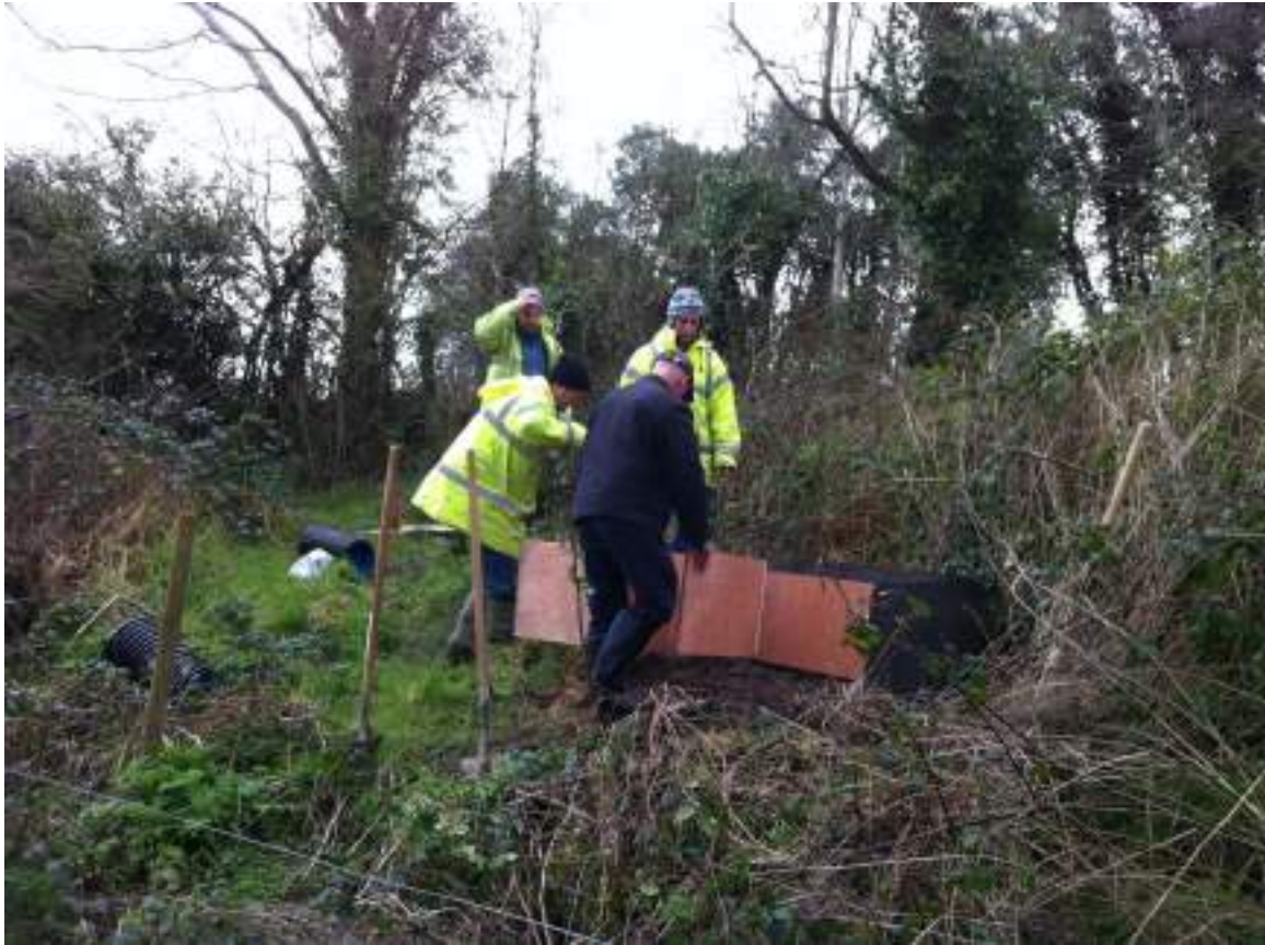
Figure 4 RSS participants installing a holt at one of the sites in Curragh, along the Dalua
