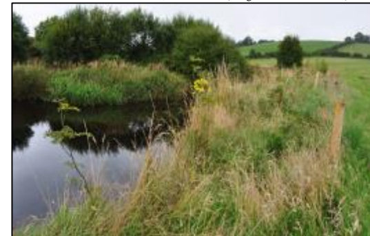
Work to stabilise bank erosion and enhance the riparian zone (Image: RÓC)
